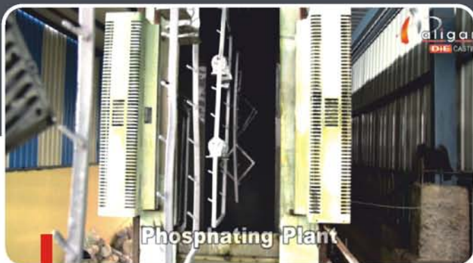
PRE-TREATMENT / PHOSPHATING PLANT
